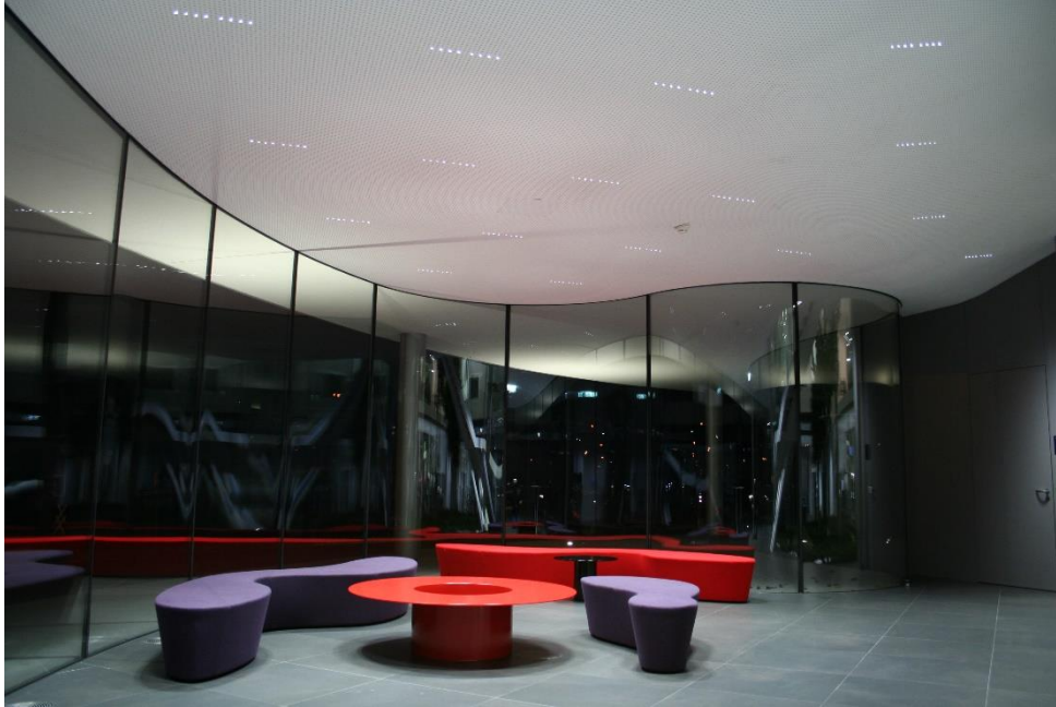
In this office building, the lens LFO is installed almost invisibly in the acoustic plasterboard ceiling. The light source does not detract from the architecture. © Bartenbach GmbH
